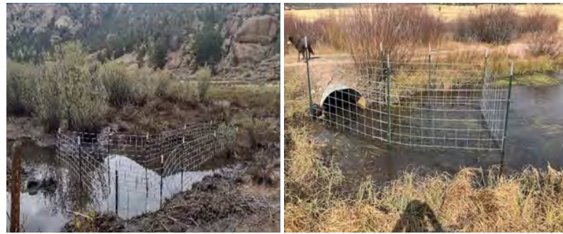
Figure 25: Exclusion fence installations are all site-specific and using the basic design principles, can be adapted by a trained professional for a variety of different waterways and needs. Photo Credit (left): Aaron Hall; Photo Credit (right): Elissa Chott.
